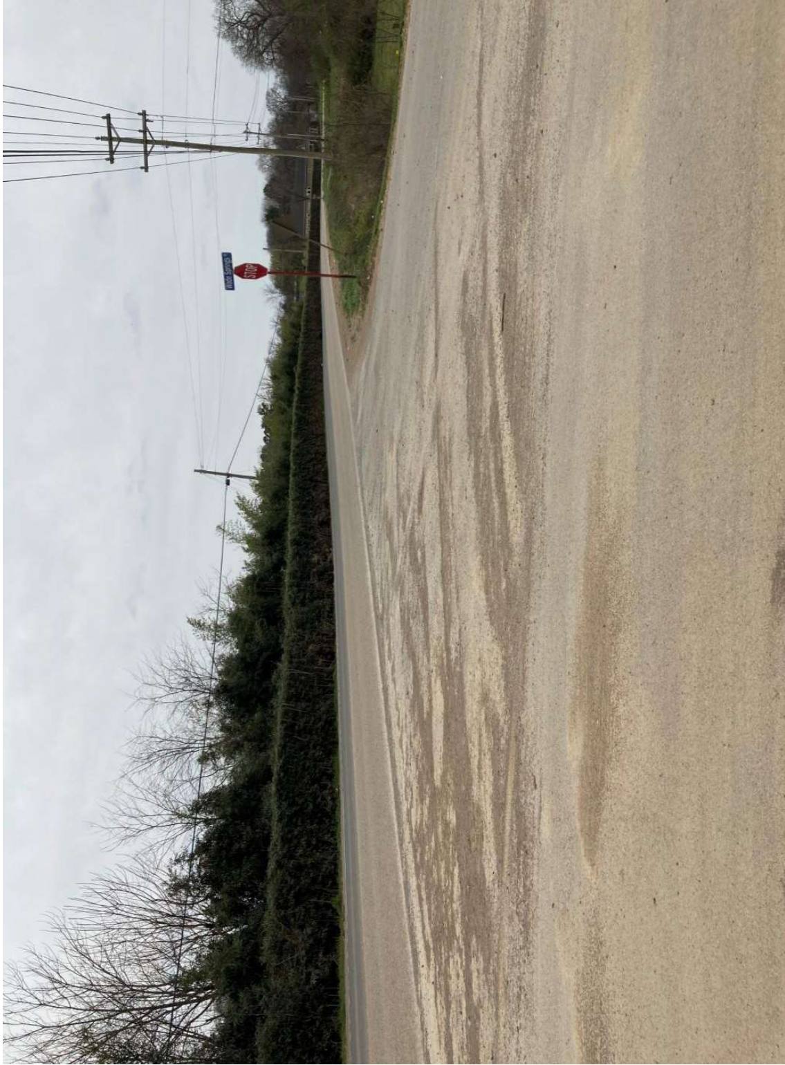
Photo 5: Sediment build up at Wade Springs Road/East Jefferson Pike 3/29/2022.
