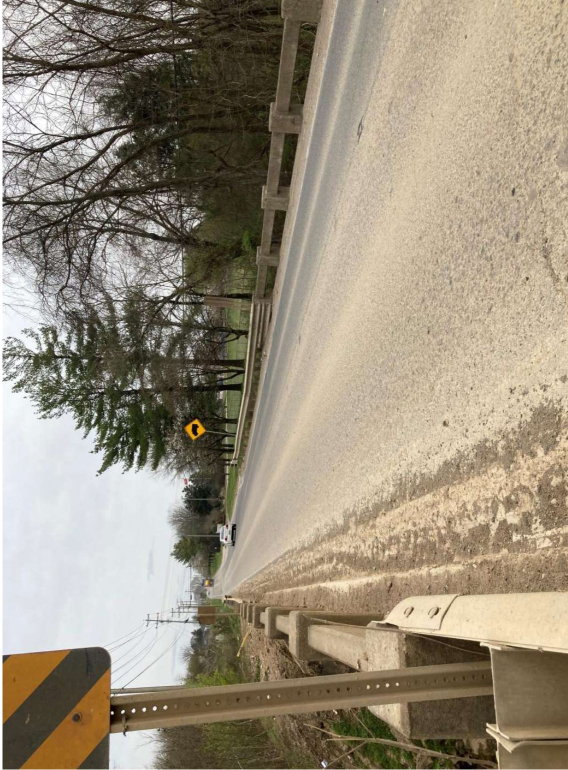
Photo 6: Sediment build up along East Jefferson Pike 3/29/2022.
